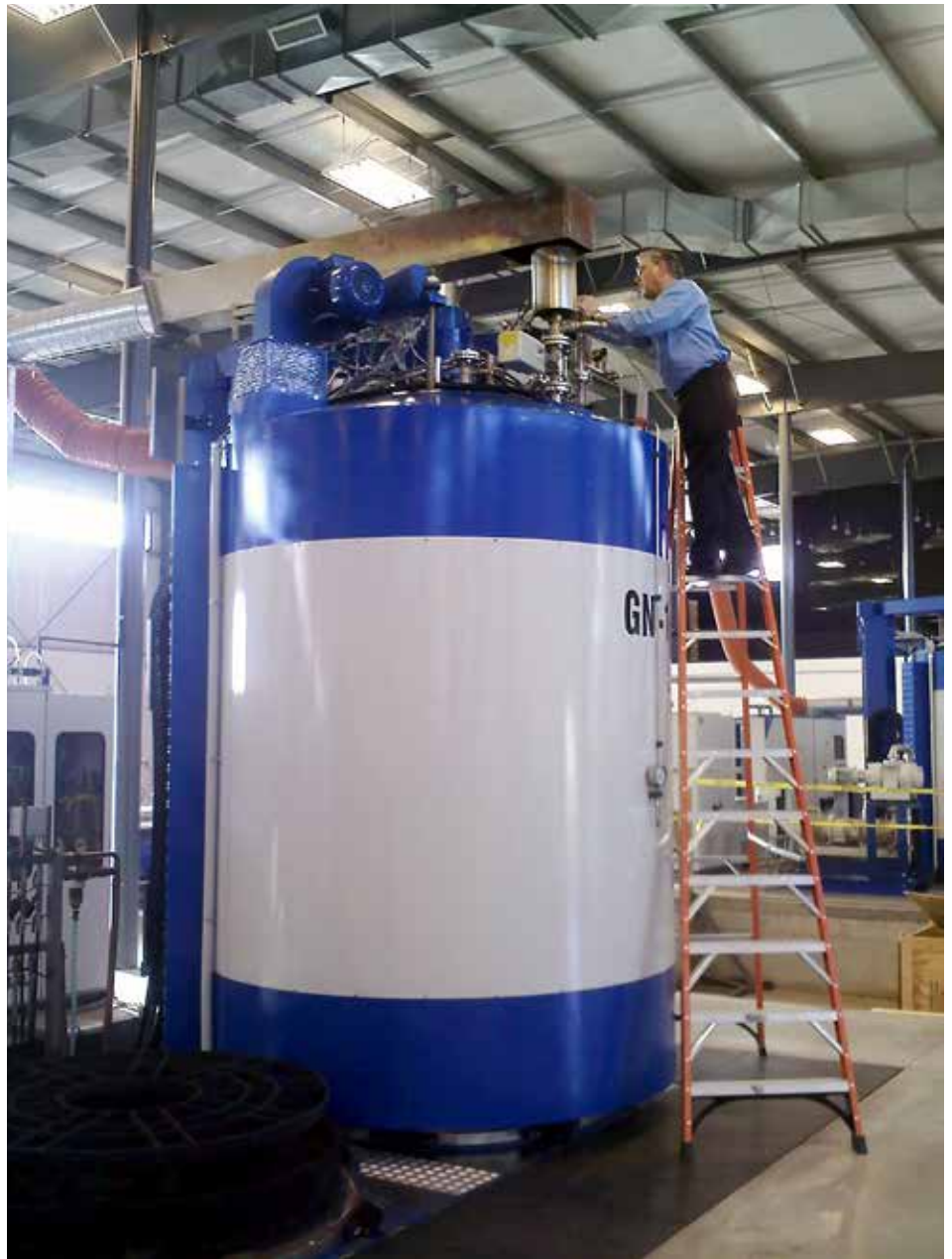
Replacing a thermocouple in the field.
